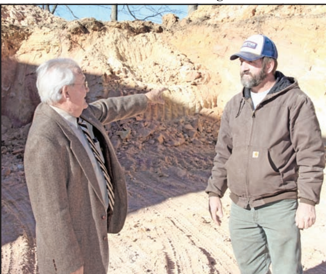
Akins discusses the ongoing construction of the showroom/storage building with Stacey Stephens of the Union County Road Department, who helped to grade the site.
